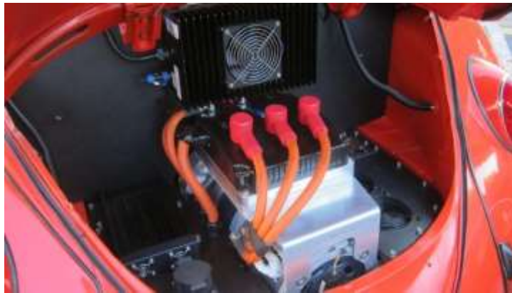
Fig. 3.4 Over 50V installation marked orange, source: www.e-auto.guru
